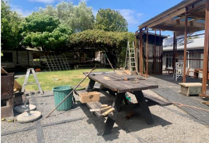
construction of the Sawmill's new pizza oven station in the garden bar
